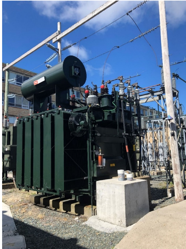
Figure 2: MUN-T2 Power Transformer
